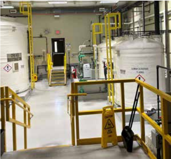
South Chemical Room
