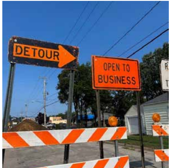
Maintaining access for residents and businesses and creating a safe construction site has been a priority from design through construction.
