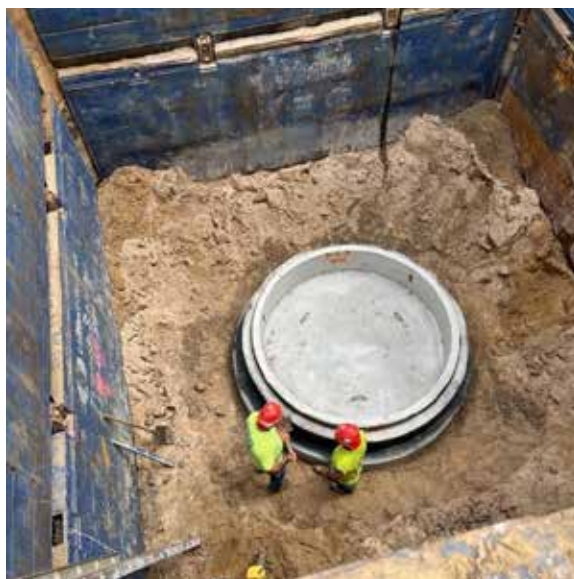
This slide rail shoring system was used to install the lift station wet well.
