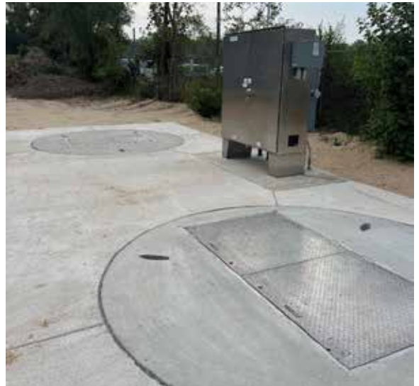
The new, recently completed lift station.
